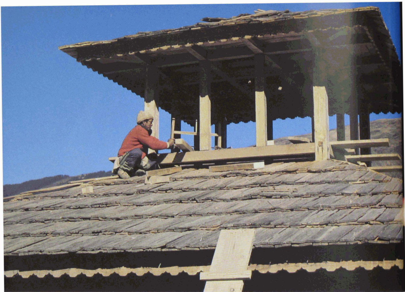
12 Tapkhay's brother working on the roof of the new gompa in Thumbuk.
